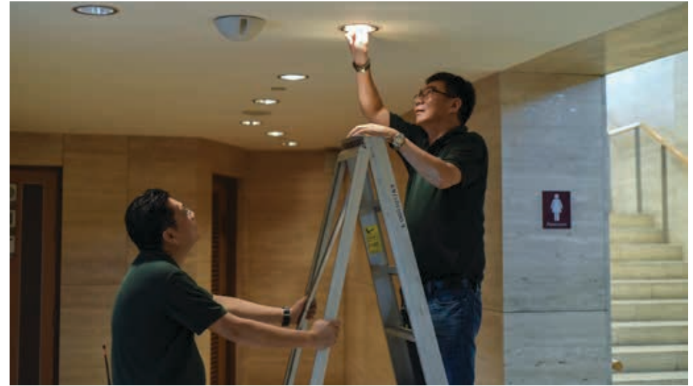
A rigorous maintenance schedule helps to ensure that the centre's systems operate optimally.
