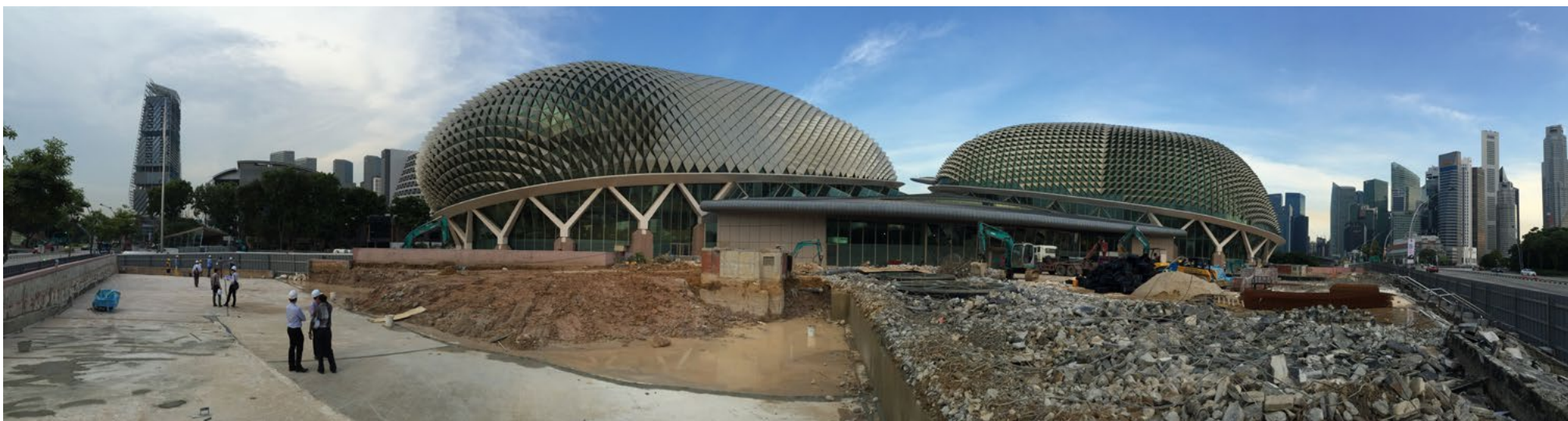
Ongoing works at the Esplanade Forecourt under Phase 2 of our A&A works.
